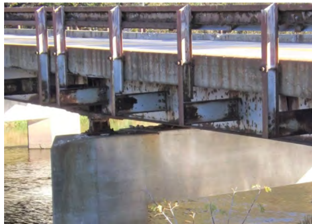
Figure 4.1 Metallic Corrosion on a Bridge, Culvert, and Motor Vehicle
