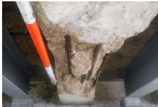
Figure 4.5 Reinforced Concrete Beam Damaged by Rebar Corrosion
