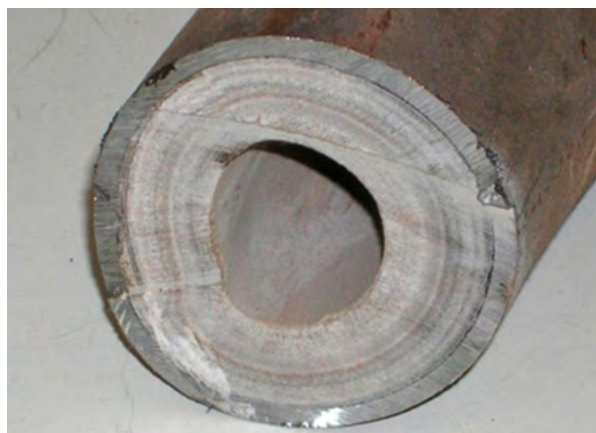
Figure: 5.1 Scale Build-up in a Water Pipe
