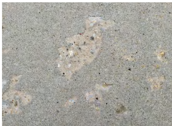
Figure 4.3 Concrete Scaling Damage
