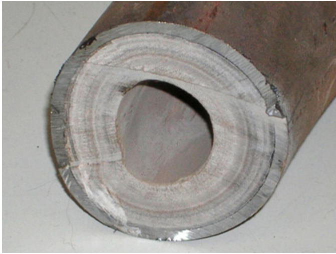
Figure 3.10 Scale Build-Up in a Water Pipe
