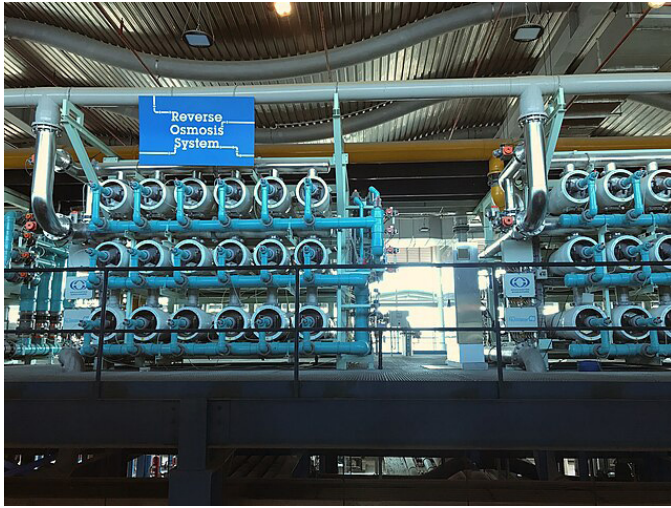
Figure 3.7 Reverse Osmosis Plant
