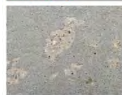
Figure 4.3 Concrete Scaling Damage
