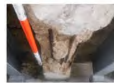
Figure 4.5 Reinforced Concrete Beam Damaged by Rebar Corrosion
