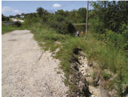
17 - EROSION AT CTH ES
