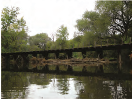
1 - WOOD DEBRIS JAM AT RAILROAD BRIDGE
